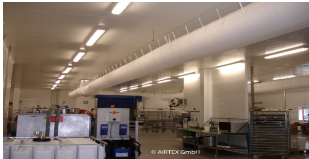
Textile ventilation ductwork Airtex Bioactive in the production unit of a wholesale bakery Photo: Airtex GmbH Textiler Luftkanal Airtex Bioactive in der Fertigung einer Großbäckerei Photo: Airtex GmbH
